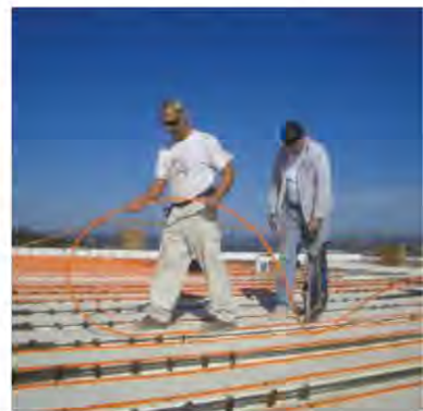
Techs from Alhadeff and Nikiforuk lay out a few of the home's 9,000 feet of PEX tubing. Rachel Wenger photo.
